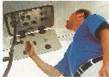
İçme suyu servis paneli
